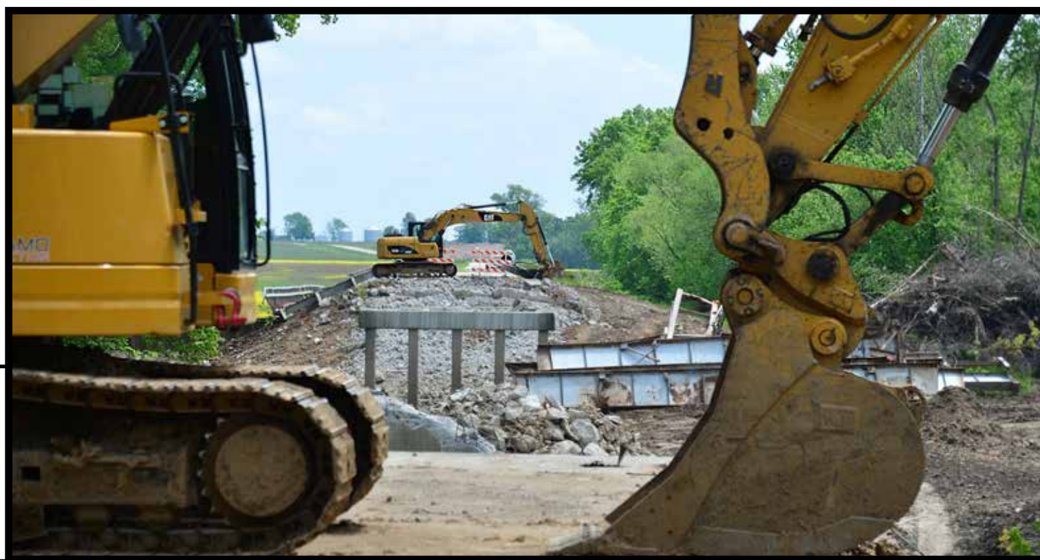
Where there was once a bridge, now is just two masses of land divided by a river with construction work rapidly moving ahead on the bridge leading east out of Louisville. (John Bayler Photo)
